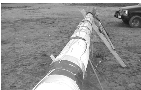
Figure 28. Trial 5 assembly of 127-mm star shells aligned with and ready to be pulled into pipe.
