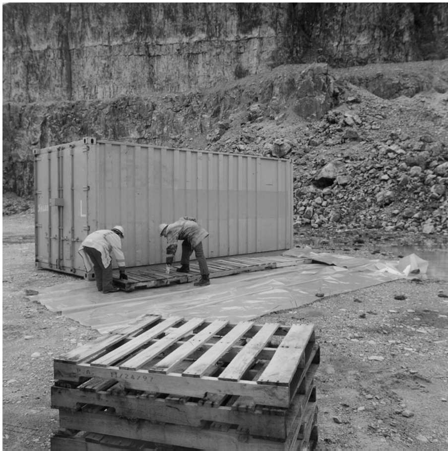
Figure 1. 6.1 m long ISO transport container.
